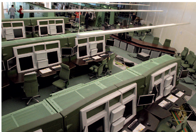
Work underway installing the Pegasus_21 system at Warsaw (photograph courtesy of Sebastian Elijasz)
