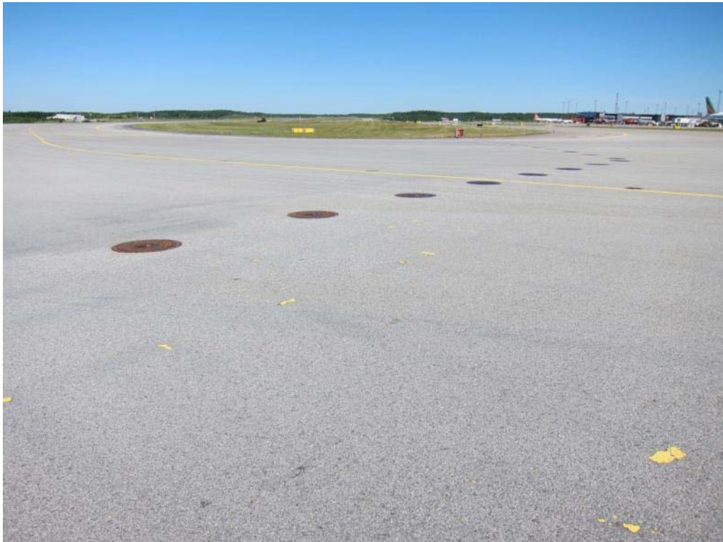
Fig. 4 Remains of previous holding position markings at Y3, 29 June 2011
