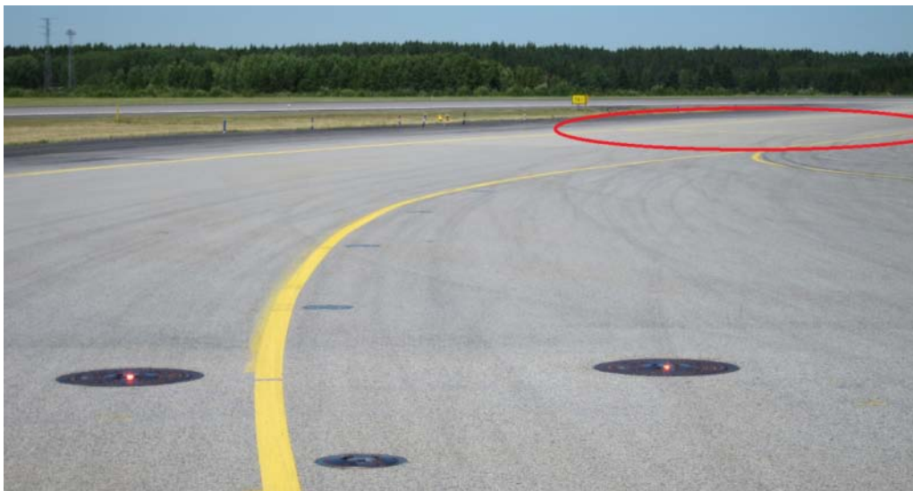
Fig. 6 Photograph taken from the holding position at Y3 in level with the stop bar, with the yellow holding position markings at the RGL circled in red, 29 June 2011.
