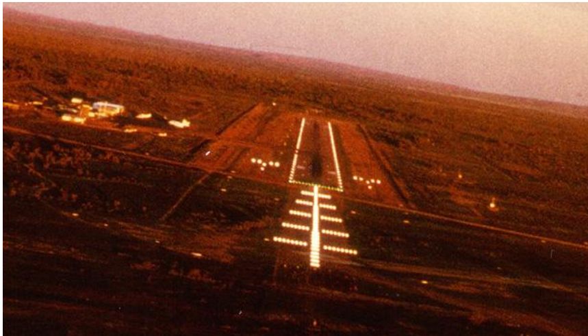
(Calvert lighting system)
