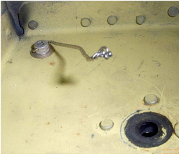
Figure 2. Lockwire on the rudder's hinge bolt
