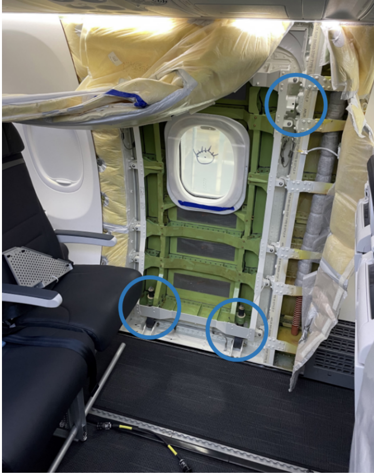
Figure 16. Photo showing the left MED plug immediately before interior restoration and the circles show the three locations without the retaining bolts, two vertical movement arrestor bolts and the forward upper guide track bolt. The aft upper guide track is covered with insulation and cannot be seen in the photo. (Source: Boeing. Image Copyright © Boeing. Reproduced with permission.)
