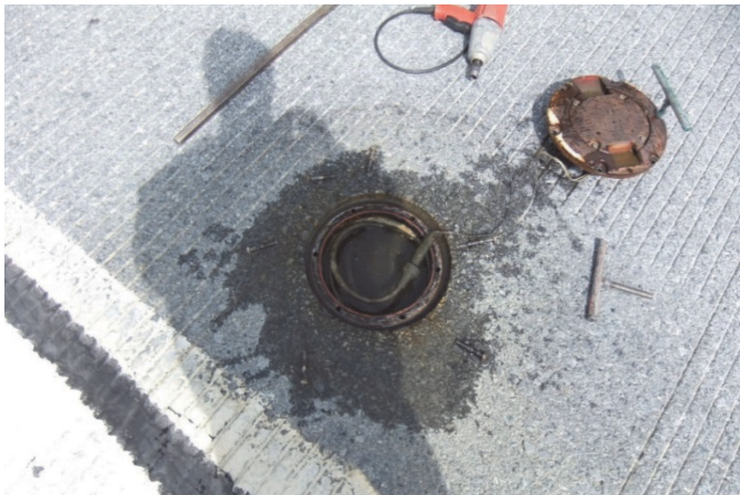
Figure 22. Water surging through lighting infrastructure.
