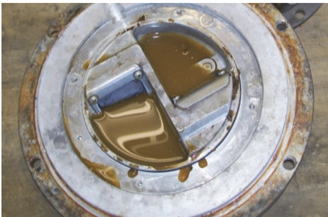
Figure 26. Water inside light fixture.
