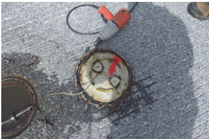
Figure 23. Primary cabling flooded by storm water.
