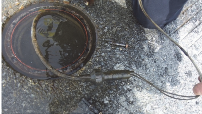
Figure 24. Accumulation of silt and corrosion on cabling.
