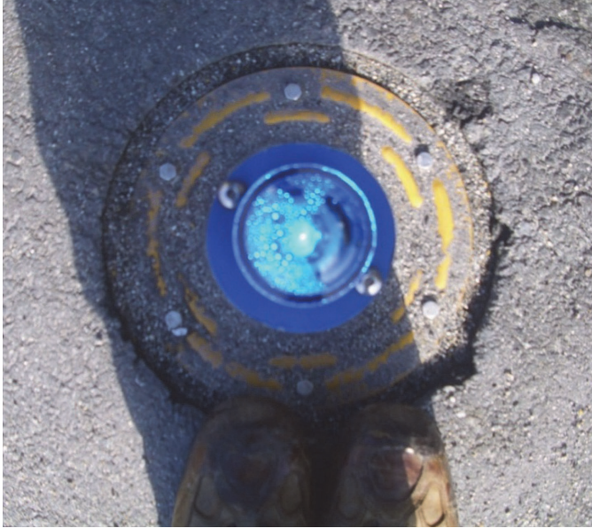
Figure 25. Moisture build-up inside fixture.
