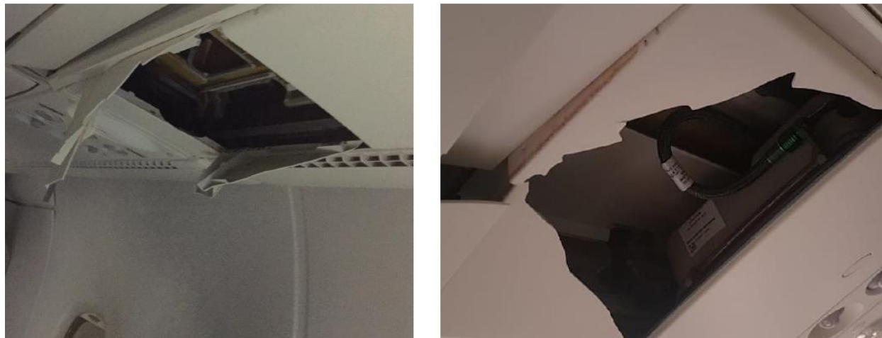
Figure 2. Main deck aft cabin ceiling panel damage
